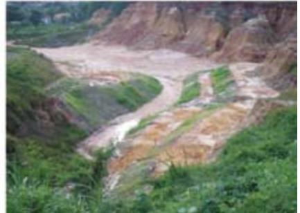
Partial view of the rehabilitation gully with grass cover, one month after rehabilitation work.
