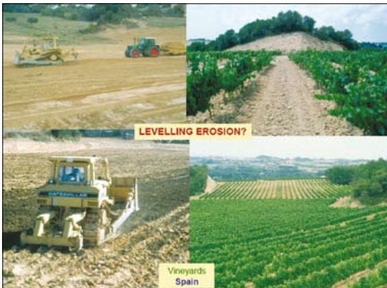
Plate 5. Examples of surface level changes in Spain.
